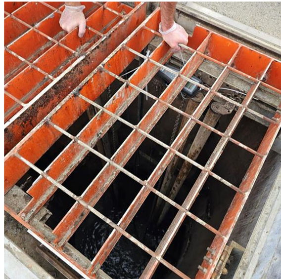
WWTP Lift Station Probe Installed
